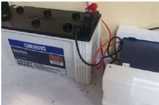
Inverter battery for power backup
